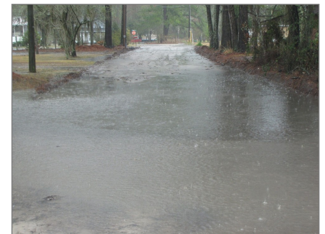
Seen above is one of the streets that will be improved with CDBG funds in Echols County. Upon completion of the project, residents will no longer be endangered by these flooded roads.
