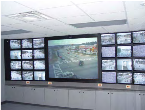
Figure 13 Valdosta Traffic Management Center Control Room
